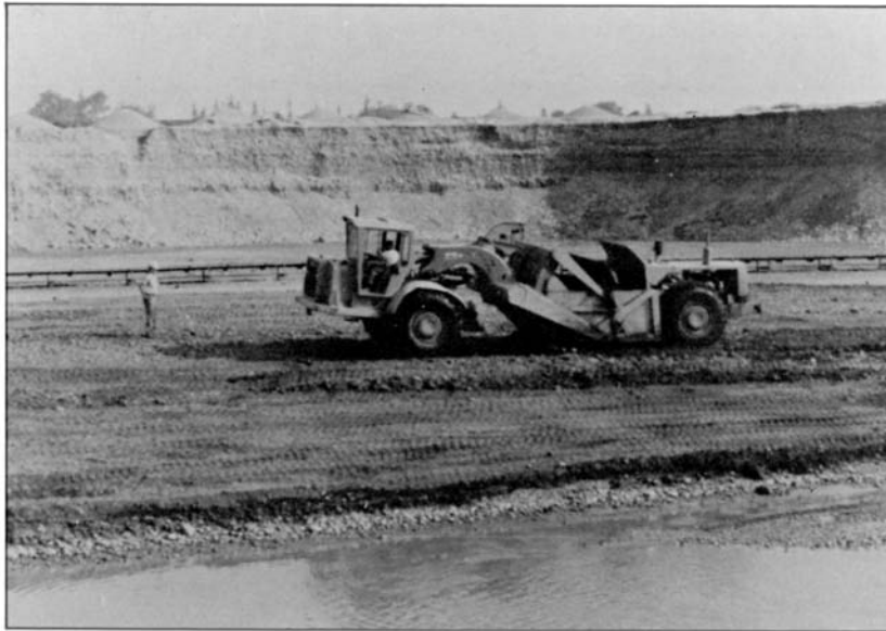
Heavy earth-moving equipment causes severe soil compaction and should not be used for reapplication of topsoil, subsoil or overburden. This earth mover can exert pressures greater than 5 kg/cm 2 when fully loaded.
