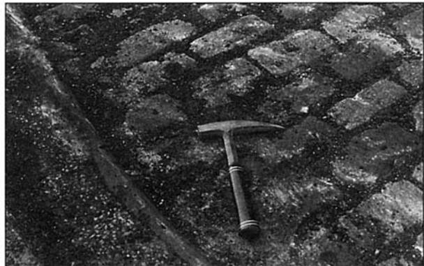
Photograph 1 Granite bricks were once a very popular road building material. In the reconstruction of Bloor Street in 1978, a layer of these bricks was uncovered as part of the old road base.
