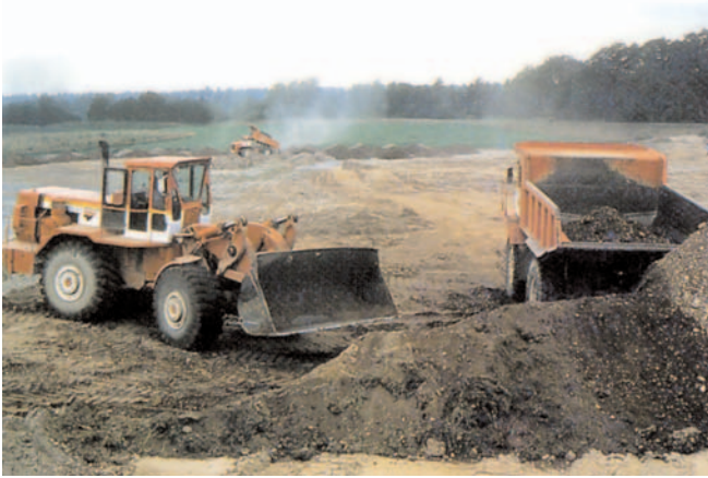
Figure 7. Where possible, topsoil and subsoil are stored separately, then replaced in order after the final pit contours are established.
