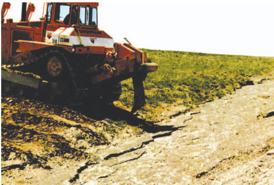
Figure 20. Subsoiling or ripping reduces soil compaction and aids in soil water infiltration and movement.
