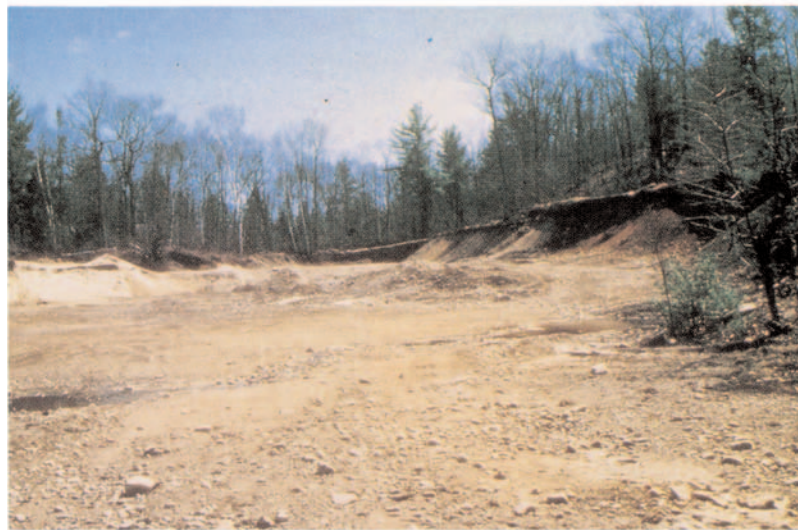
Figure 5. Illustration of conditions prior to and after rehabilitation treatment, Leslie M. Frost Natural Resources Centre, Dorset, Algonquin Region.
