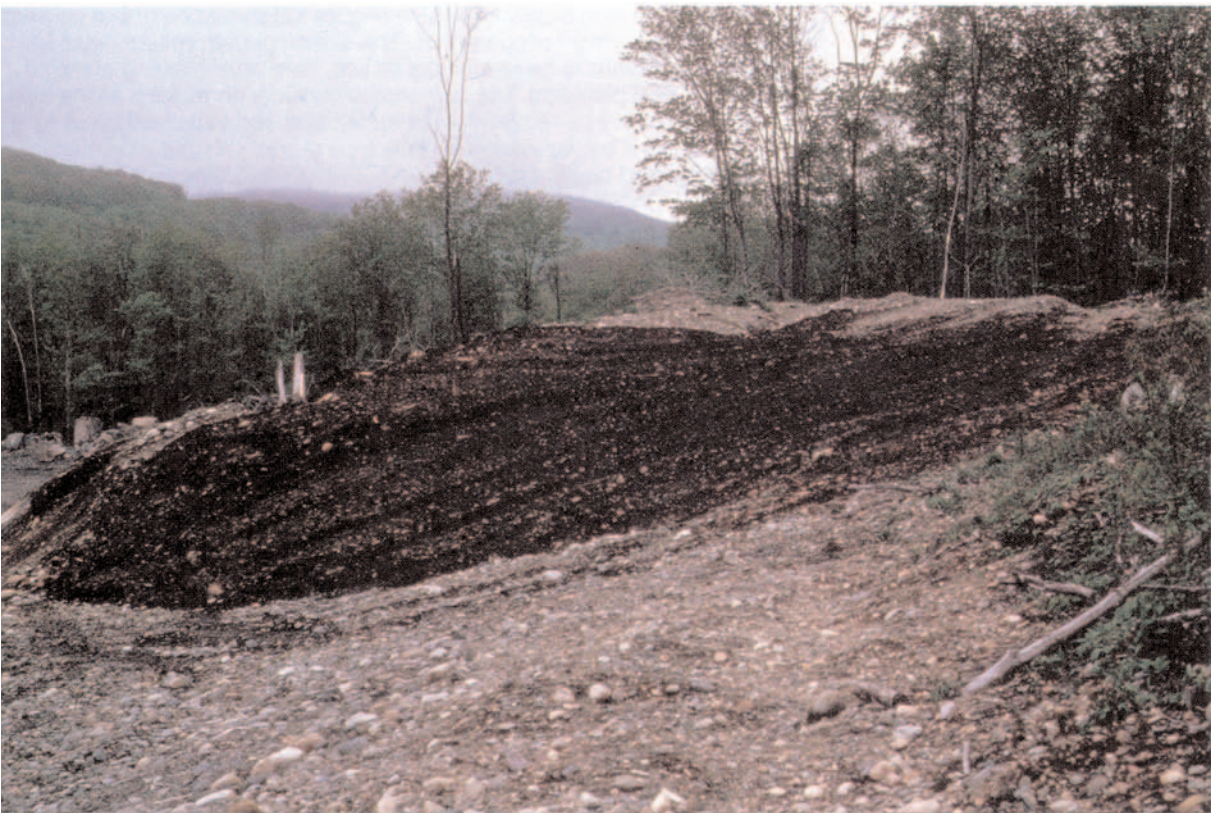
Figure 13. Once slopes have been graded and levelled, stored topsoil should be spread back over the area that is to be rehabilitated.
