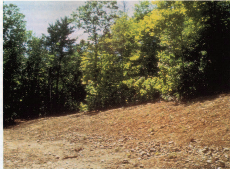
Figure 15. A slope that is properly seeded, fertilized, mulched, and planted (upper photo), will soon produce a good quality vegetation cover (lower photo).
