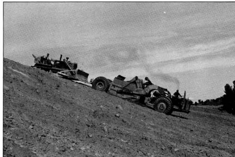
Site preparation normally involves heavy machinery for earth moving and grading. (Guelph Dolime)
