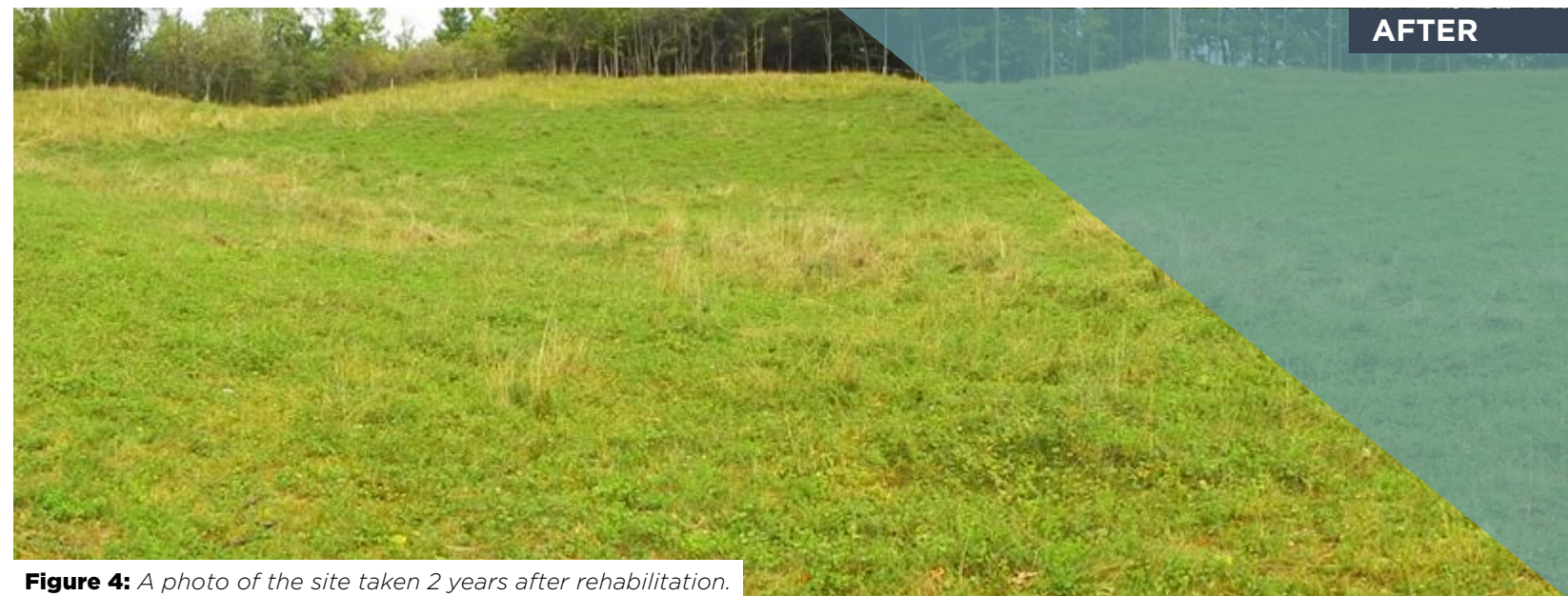
Figure 3: After the site was graded to a max slope of ~5:1 and the soil prepared for seed, the workers began the hydroseed + soil amendment application.
