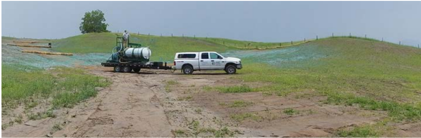
Figure 1: A truck towing a slurry of seed, ProGanics, Fertilizer and Tackifier (erosion control product) and a worker hydraulically applying over the finished grade of a legacy site.
